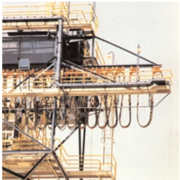
ON THE COVER: Typical Gleason I-beam festoon system providing power and control to a crane.
